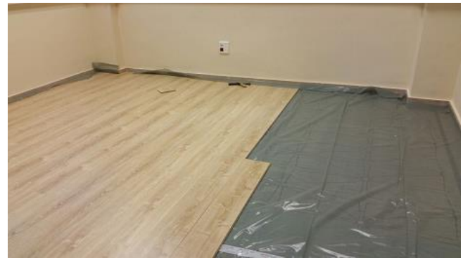
FIGURE 16. Installation of the Sensor Floor in the UJAmI Smart Lab
